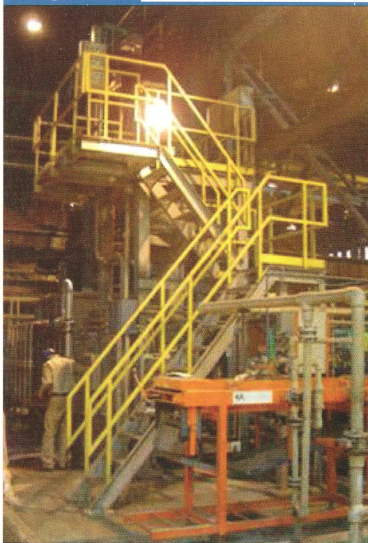
Tin dissolving plant at Ternium Siderar.
